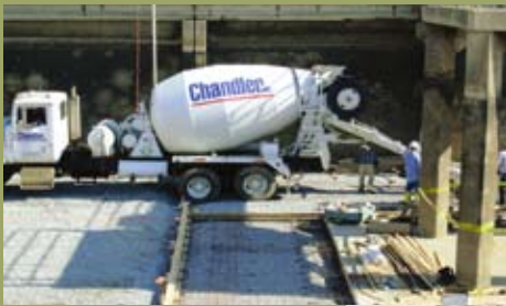
Delivering to the Waste Water Treatment plant in Salisbury
